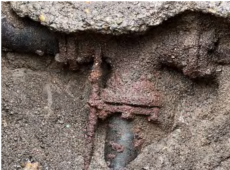
Oak Grove Apt. Existing Service Line
