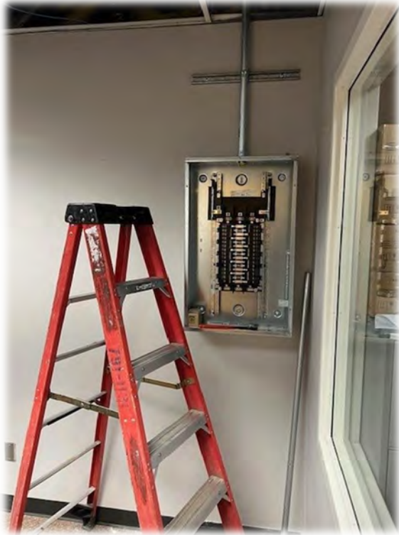
New Electrical Panel in Laundry Room
