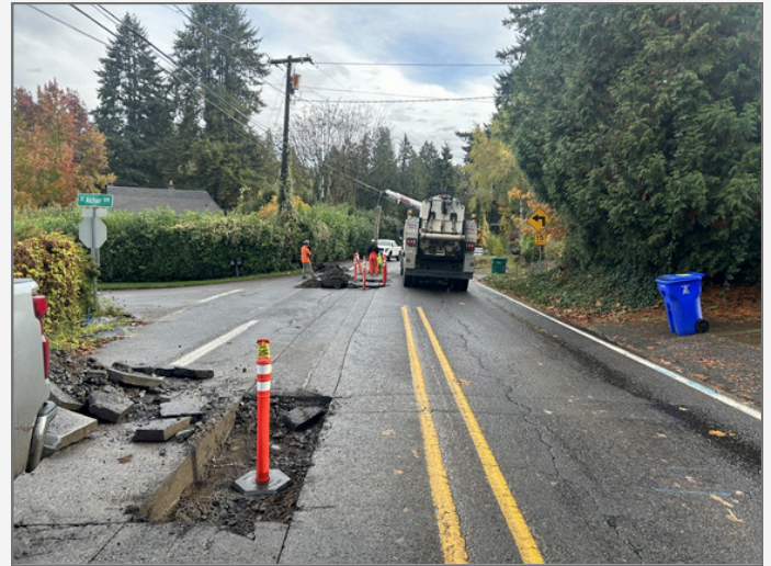
Water system improvement work on Oatfield Rd., one of the projects to be featured at this event.
