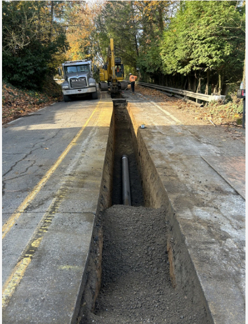
A new water main pipe is installed as part of the Oatfield Rd. project
