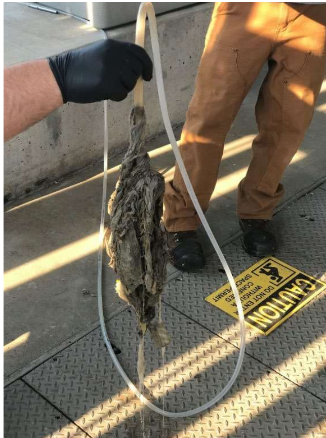
Figure 9. Debris accumulation on influent sampler suction strainer
