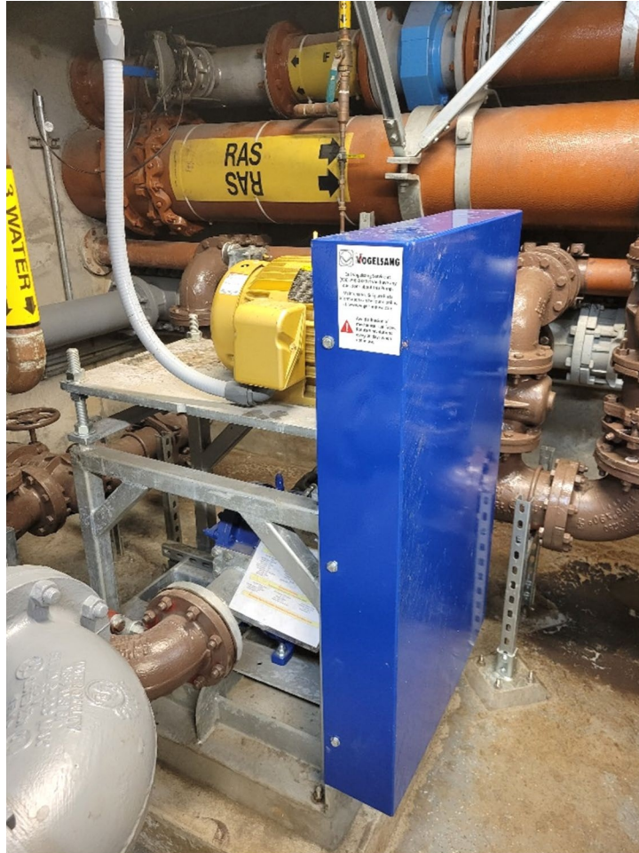
Figure 28. WAS Pump 3 in RAS/WAS pump station
