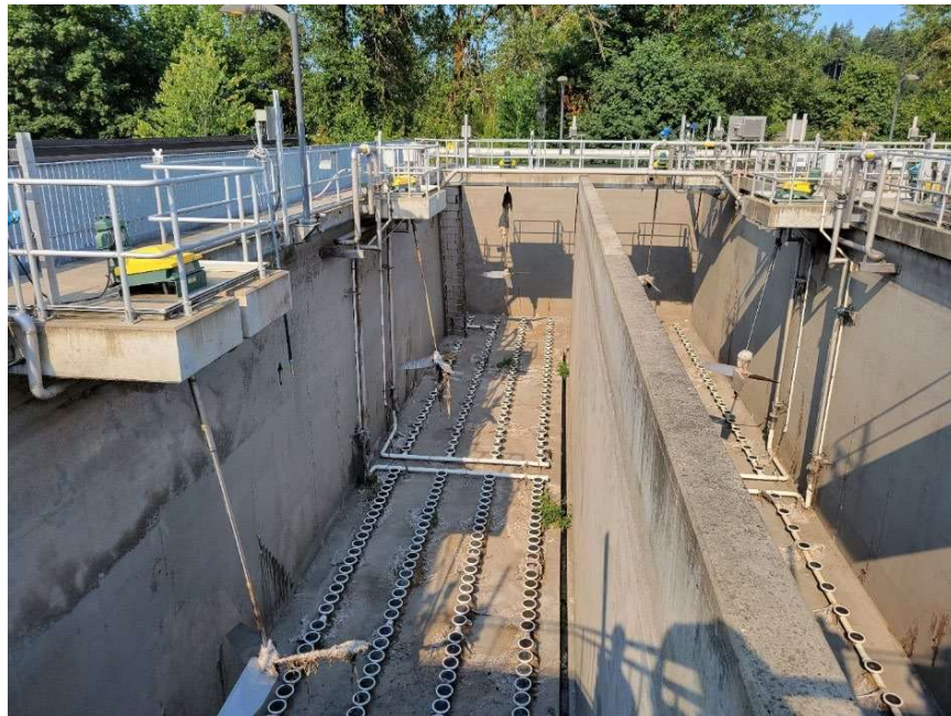
Figure 16. Aeration Basin 1 with mixers visible
