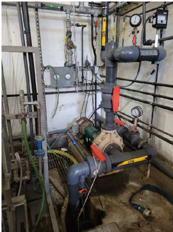
Figure 54. Chemical recirculation pump
