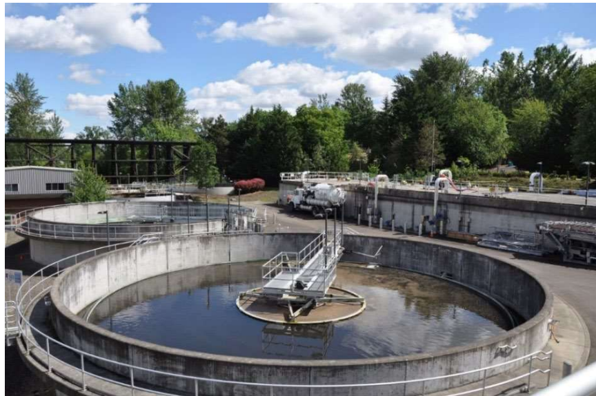
Figure 23. Newer secondary clarifier
