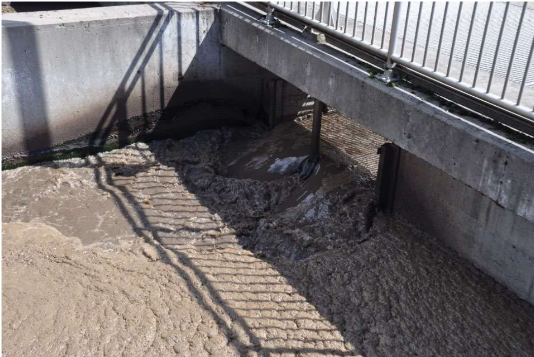
Figure 18. Hydraulic restriction at aeration basin weir gate
