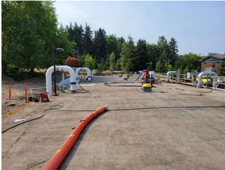
Figure 28. Top of Aerobic Digesters 1 and 2
