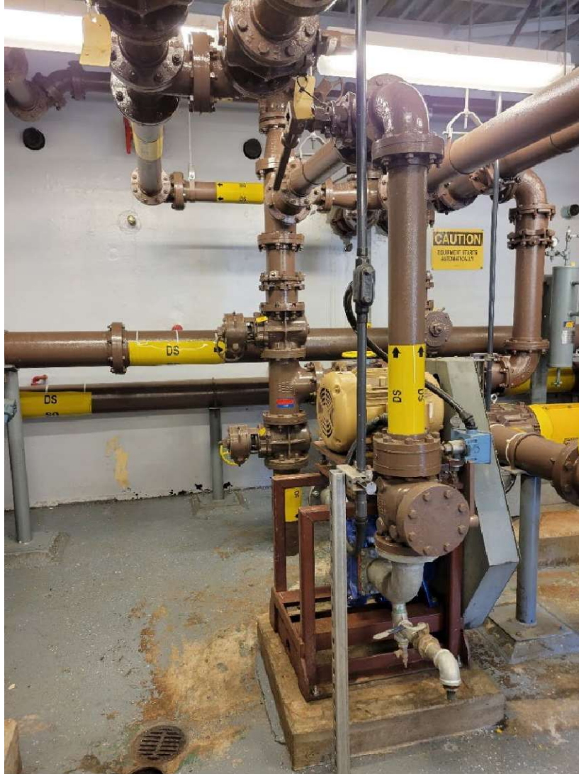
Figure 31. Digested sludge pump
