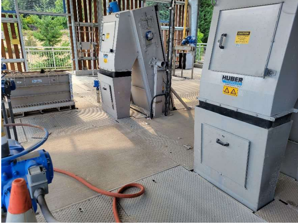
Figure 11. Multi-rake influent screens
