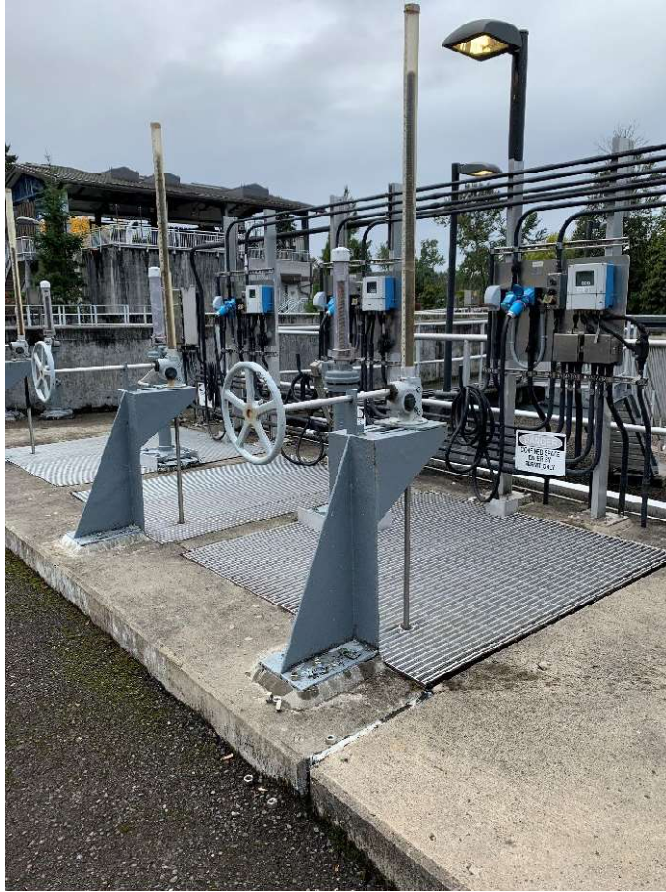
Figure 32. East RAS pumps
