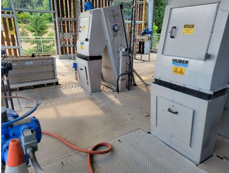
Figure 10. Multi-rake influent screens
