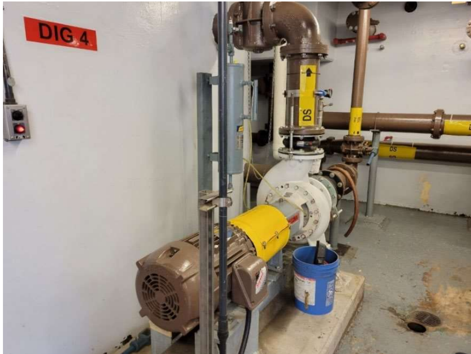
Figure 30. Digester mixing pump
