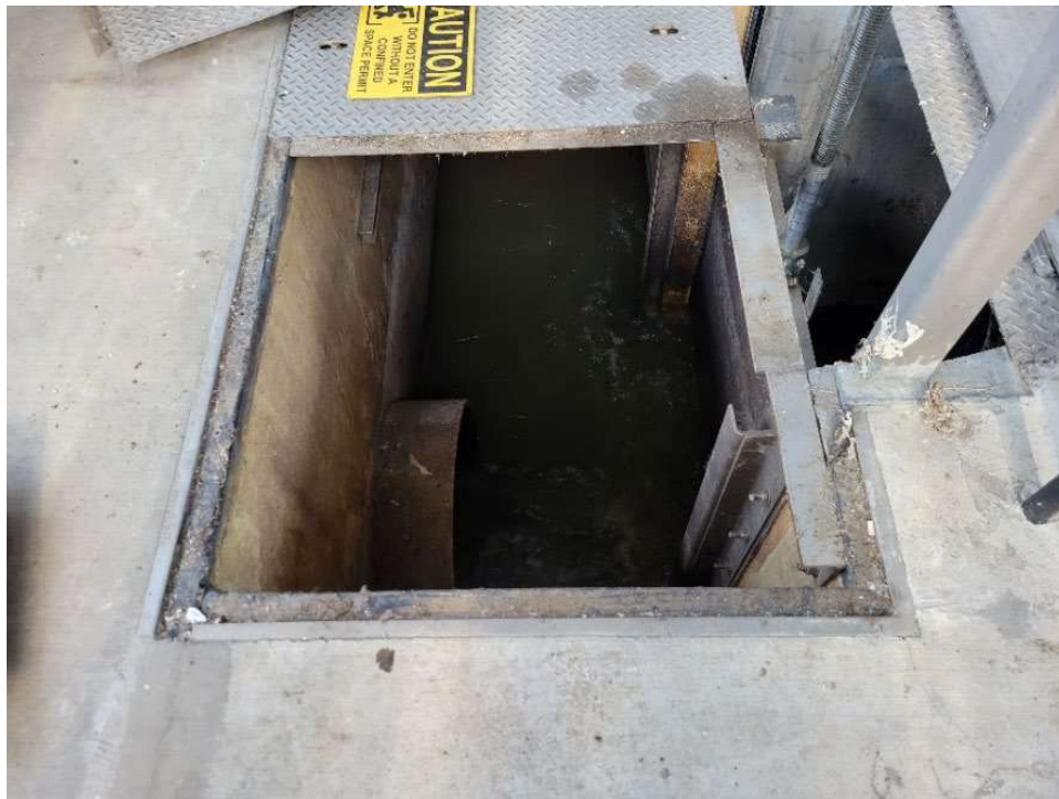
Figure 8. Raw sewage discharge into end of influent channel
