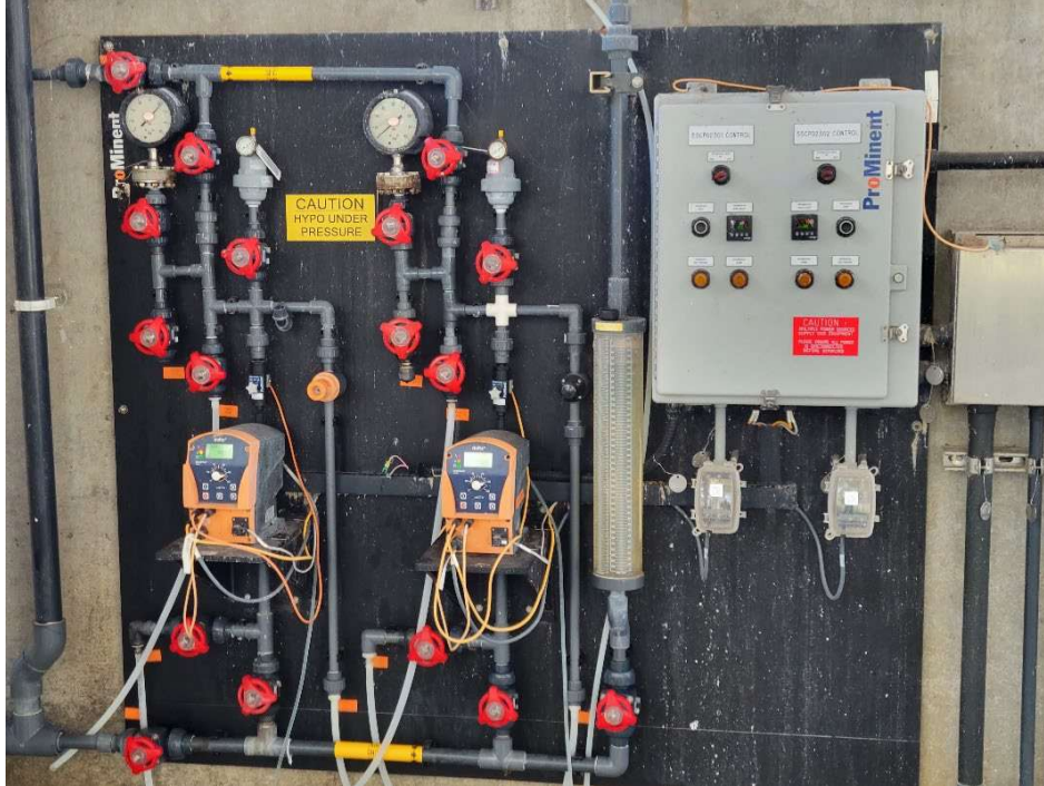
Figure 48. Sodium hypochlorite metering system
