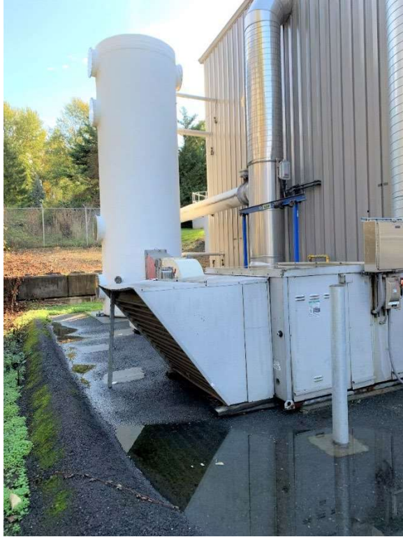
Figure 53. Chemical scrubber tower and foul air fan
