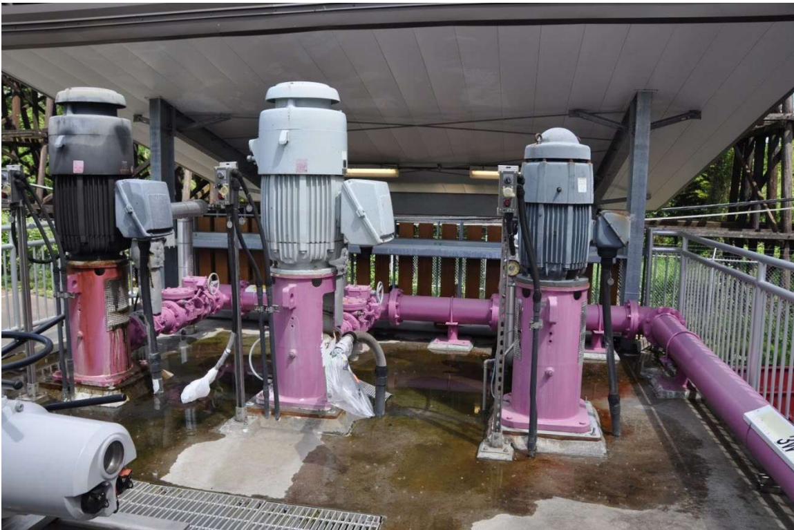
Figure 34. 3W pumps located at the disinfection facility
