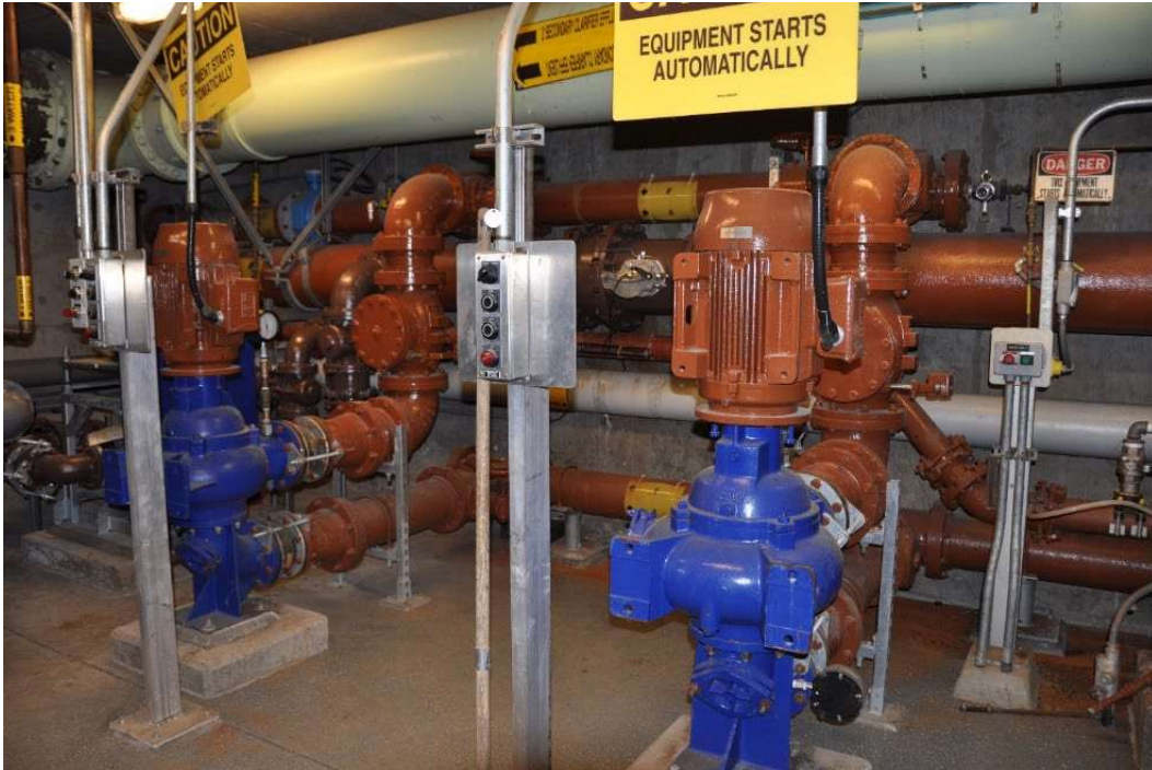
Figure 27. IBR feed pumps in RAS/WAS pump station
