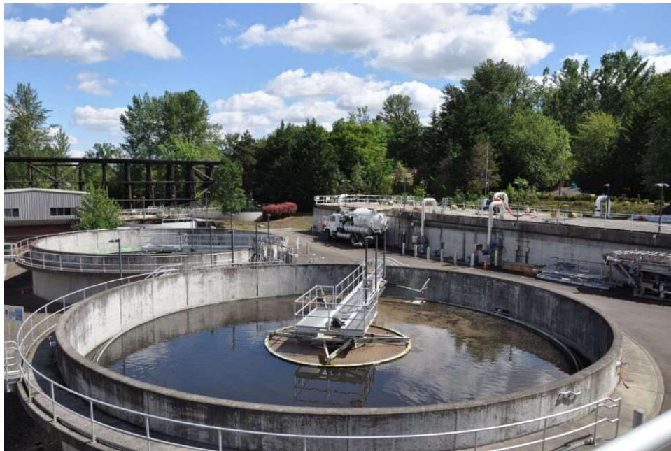
Figure 30. Newer secondary clarifier
