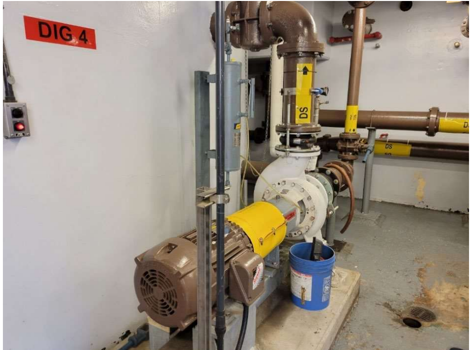
Figure 40. Digester mixing pump
