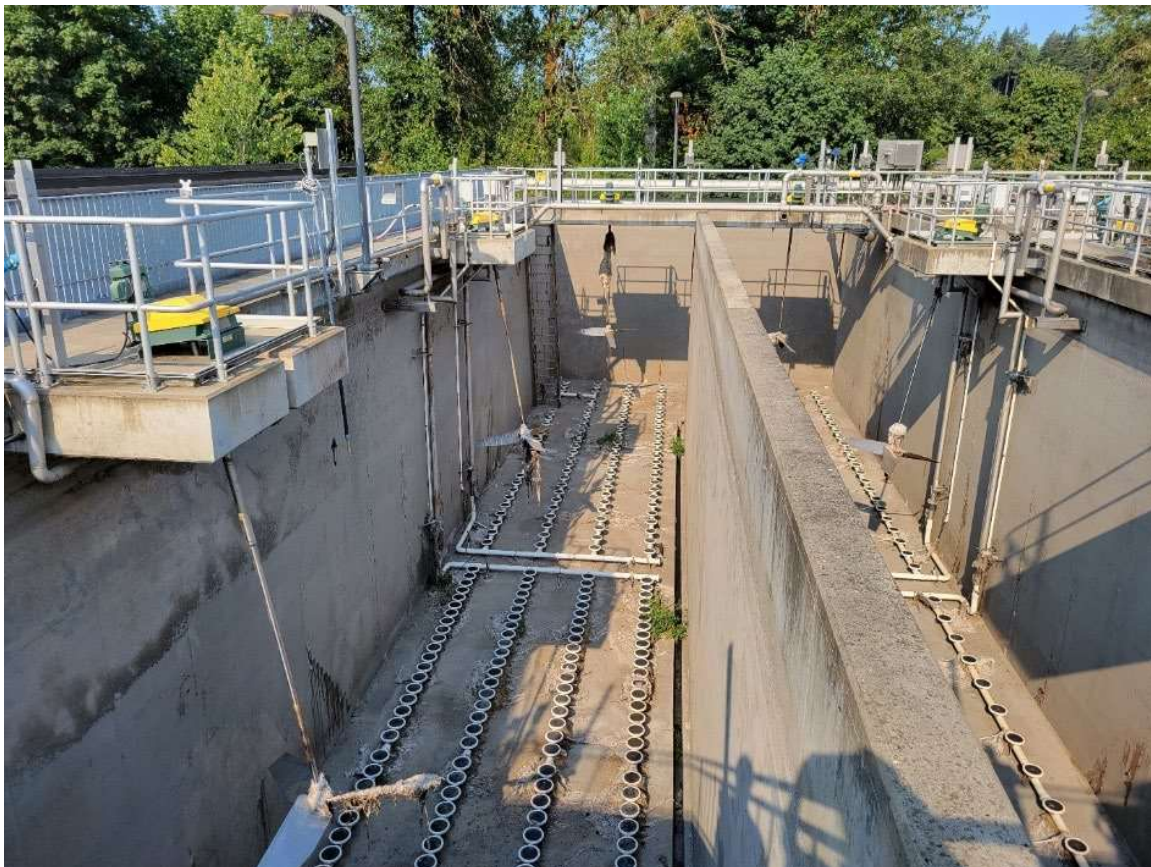
Figure 21. Aeration basin 1 with mixers and fine bubble diffusers visible
