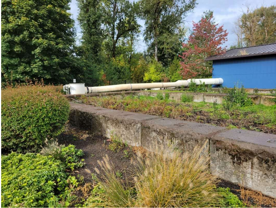
Figure 52. Biofilter building and foul air piping
