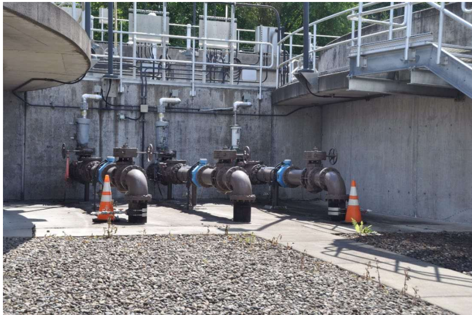
Figure 33. East RAS pump discharge
