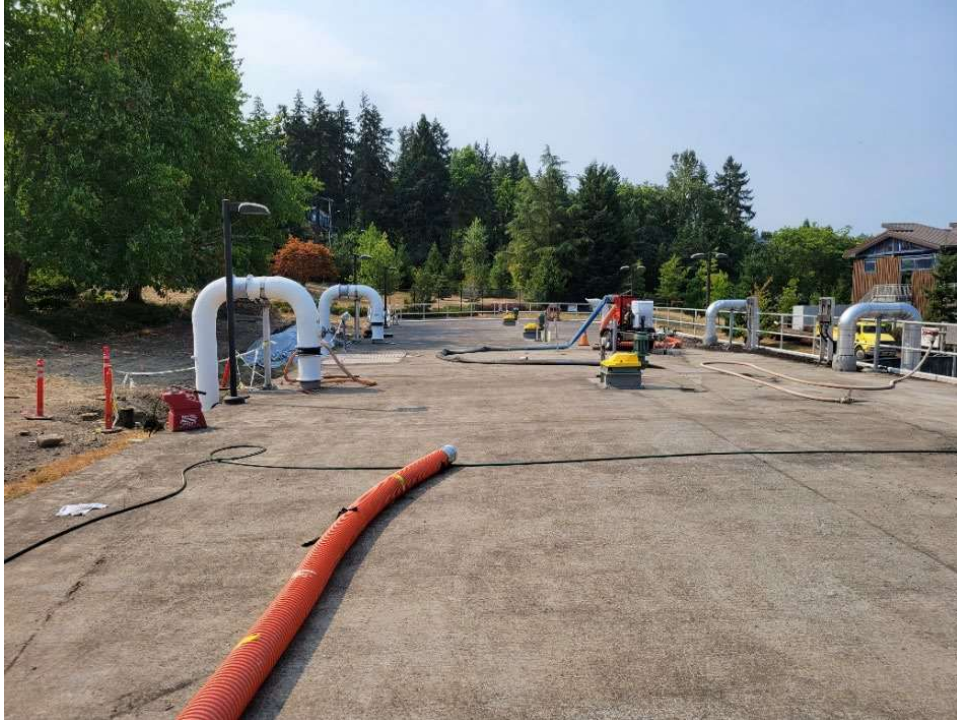
Figure 36. Top of Aerobic Digesters 1 and 2
