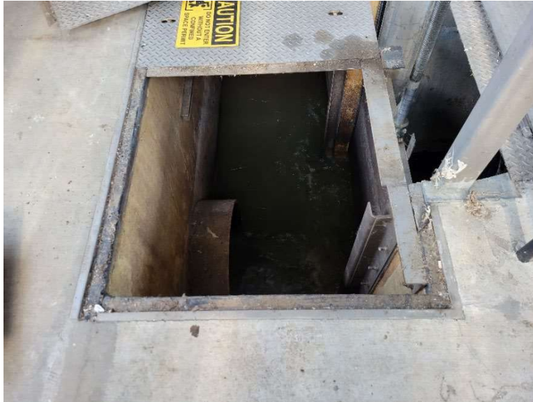
Figure 7. Raw sewage discharge into end of influent channel
