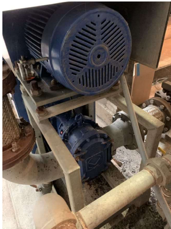
Figure 44. Thickened waste activated sludge pump
