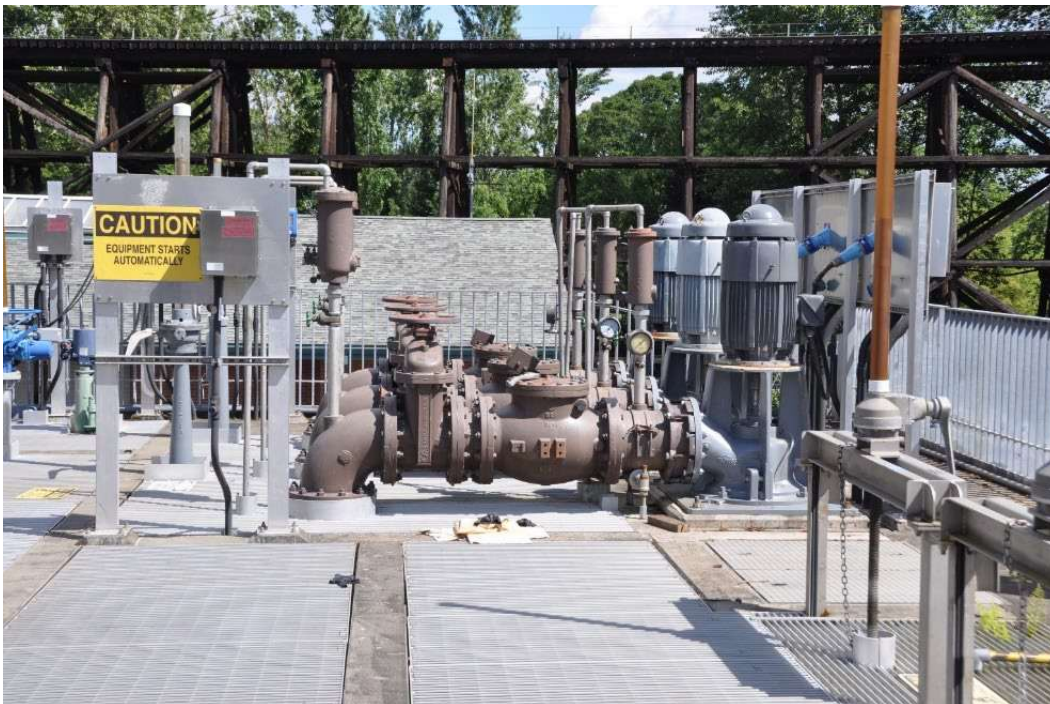
Figure 19. Internal MLR pumps
