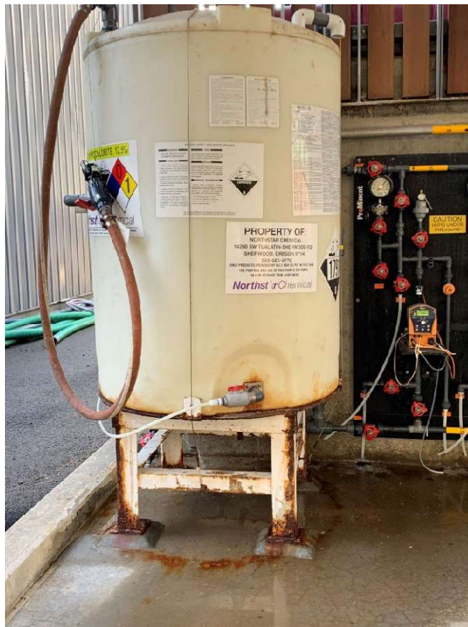
Figure 49. Sodium hypochlorite storage tank
