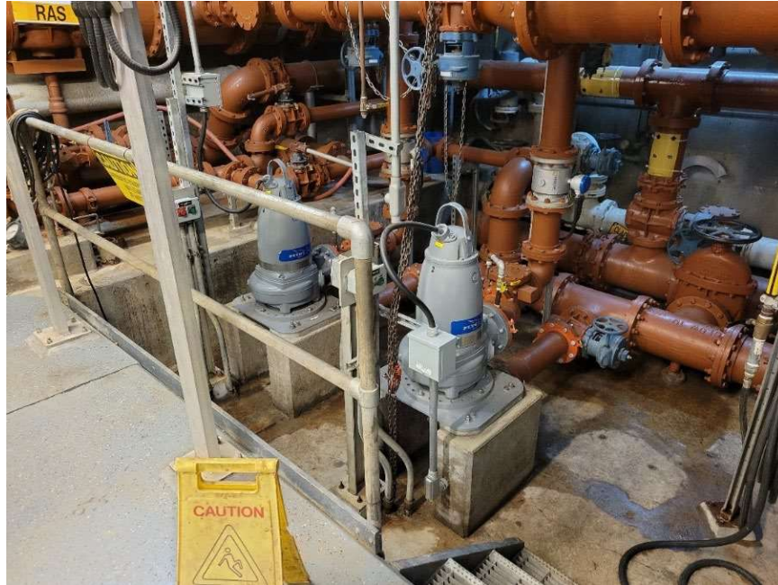
Figure 24. RAS pumps in RAS/WAS Pump Station
