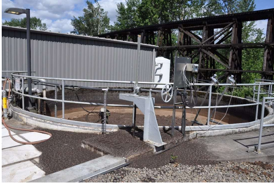
Figure 39. Circular aerobic digester
