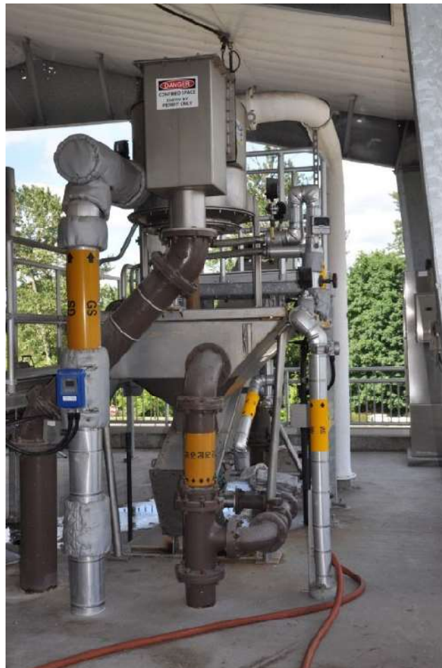
Figure 19. Grit washing and dewatering equipment
