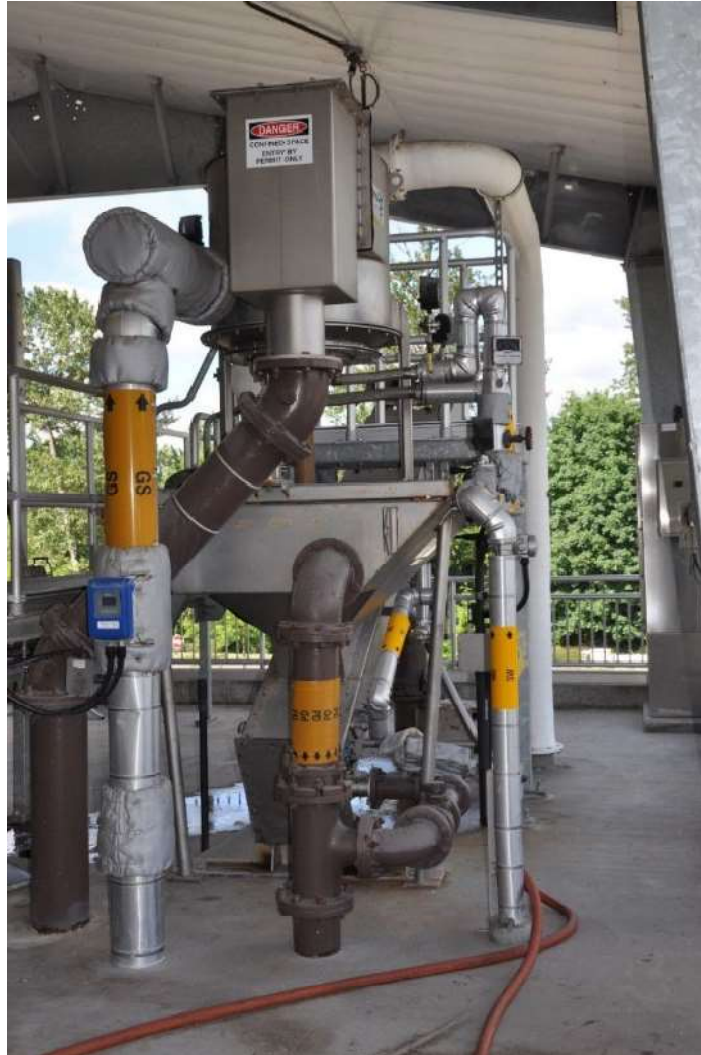
Figure 14. Grit washing and dewatering equipment
