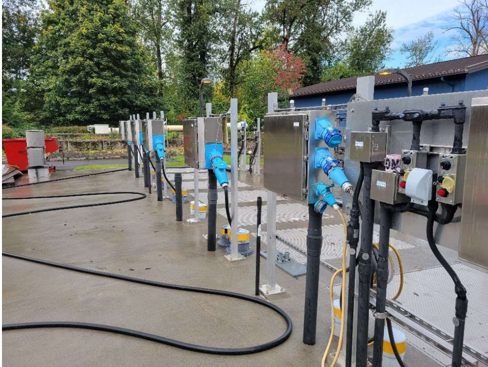
Figure 4. IPS and Plant DPS controls at grade
