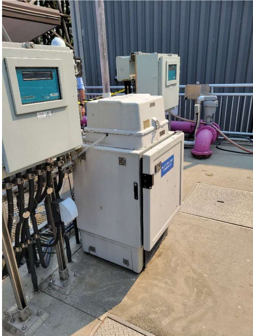
Figure 35. Effluent flow meter panels and composite sampler
