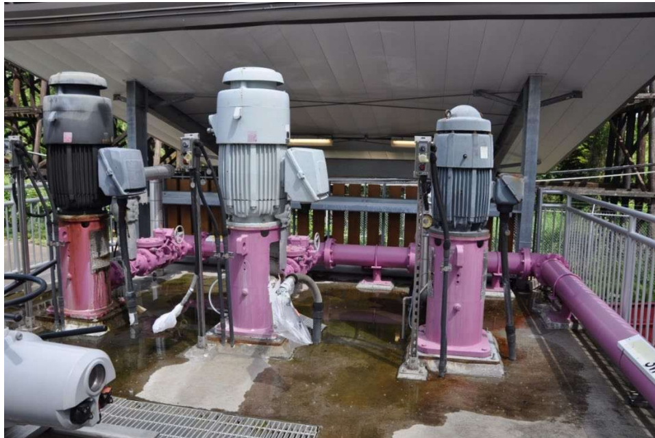
Figure 50. 3W pumps located at disinfection facility
