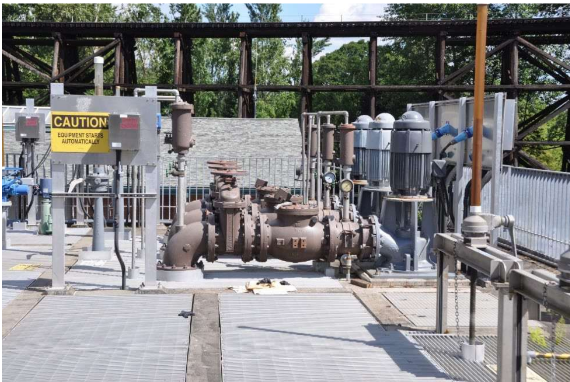
Figure 25. Internal mixed liquor recycle pumps
