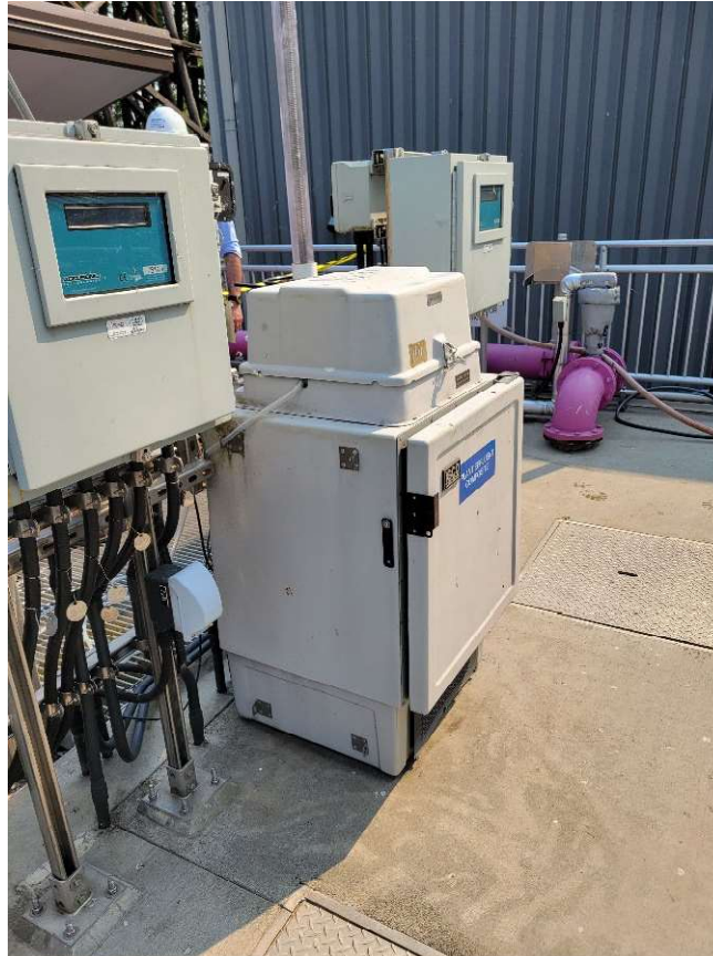
Figure 27. Effluent flow meter panels and composite sampler
