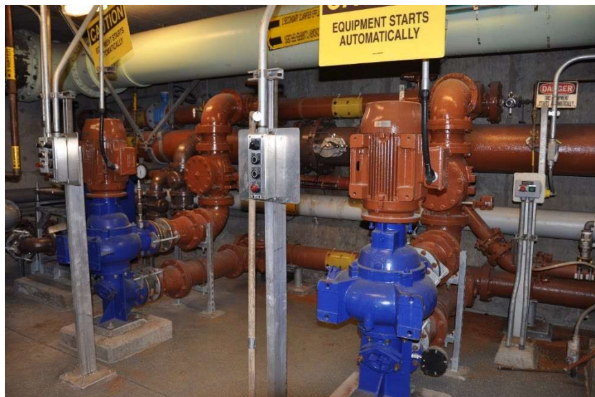
Figure 21. IBR feed pump in RAS/WAS Pump Station
