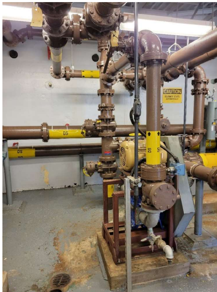
Figure 42. Digested sludge pump
