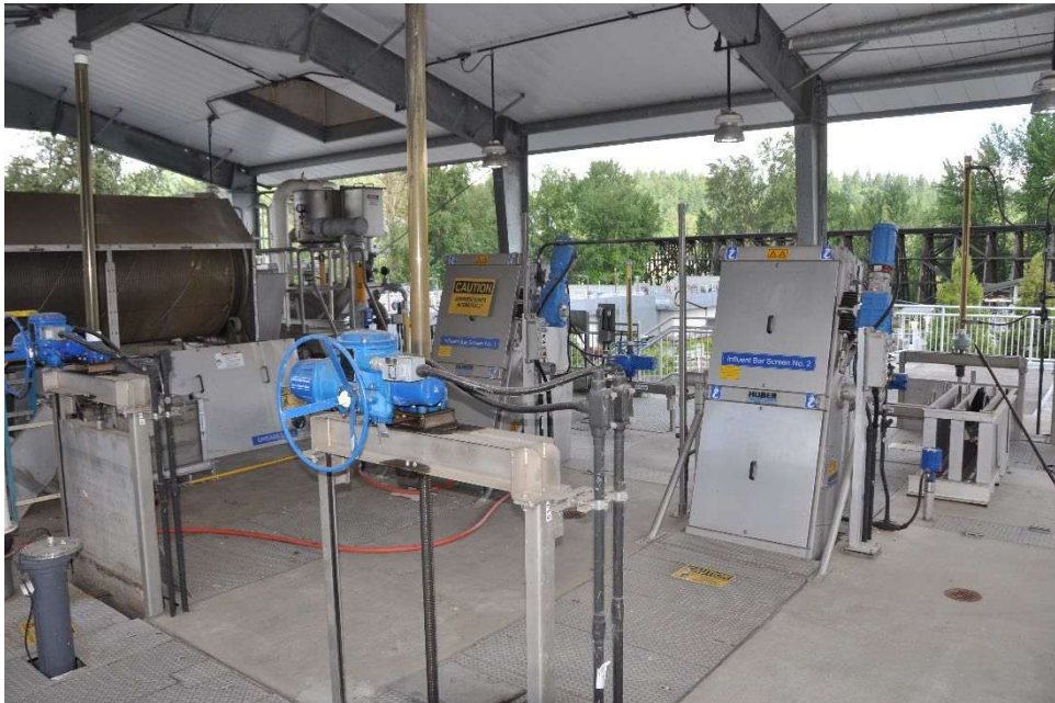
Figure 12. Influent screens with influent and effluent gates
