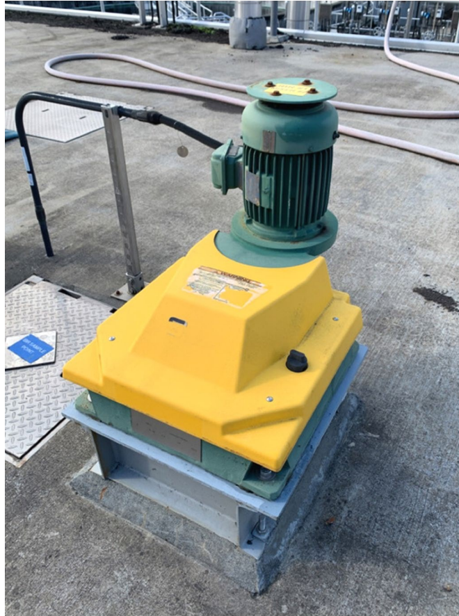
Figure 38. Aerobic Digesters 1 and 2 vertical turbine mixer motor
