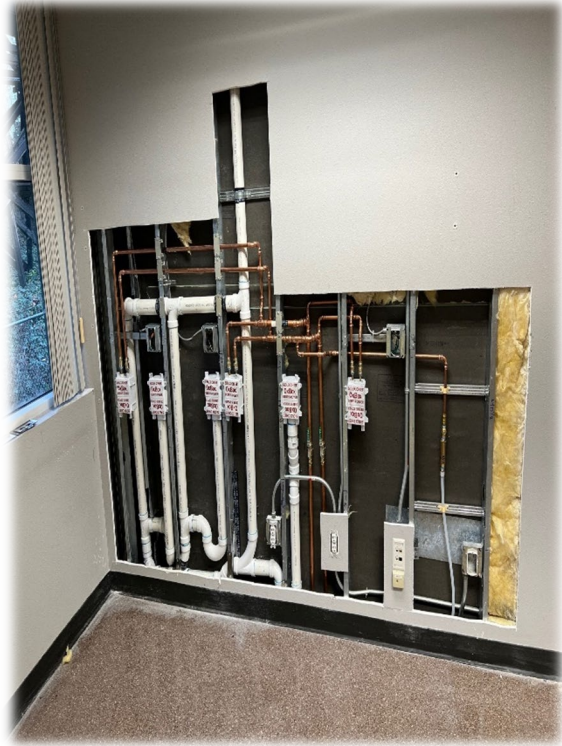
Laundry Room Plumbing and Electrical.
