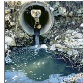
High severity suds Rating: 3 Sewage
