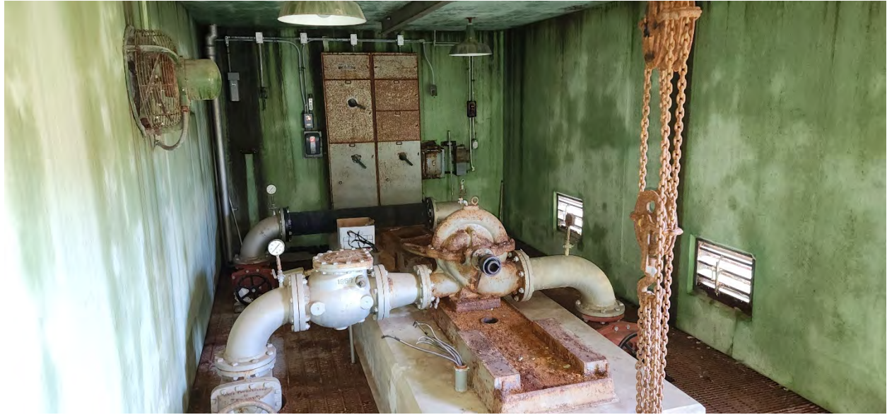
Figure F.3 – Pump Station Interior
