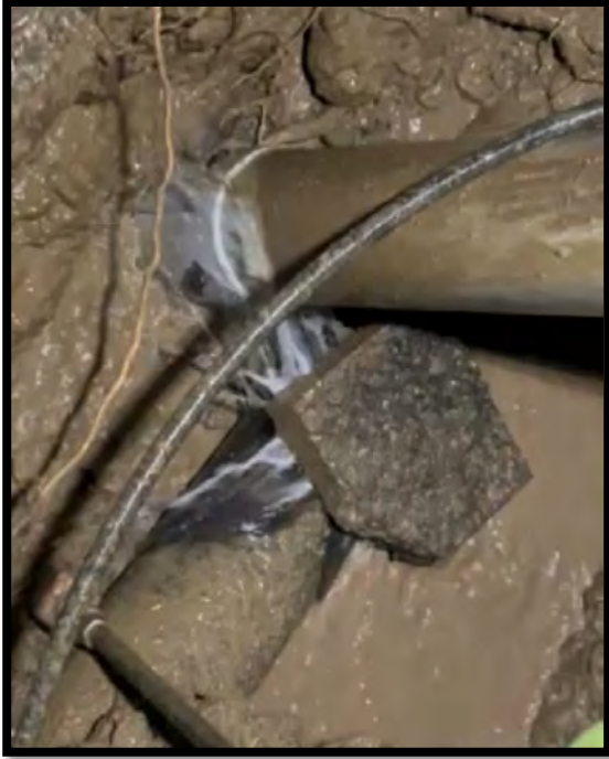
Westview Avenue Main Break
