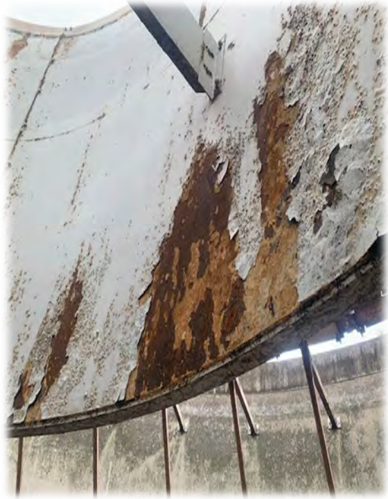
Clarifier #2 corrosion on stilling ring.
