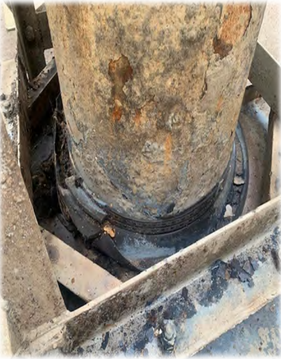
Clarifier #2 corrosion on center mechanism.
