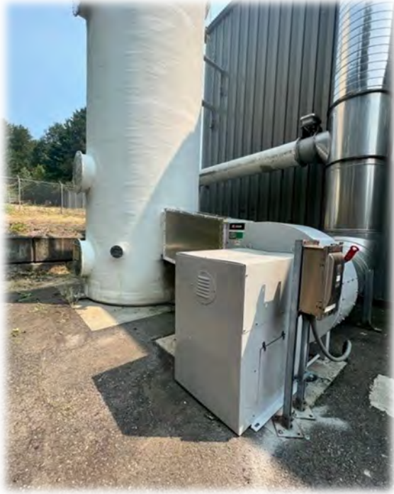
Another angle of the odor control fan.
