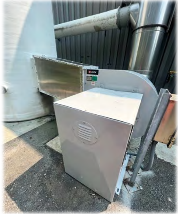
Close up of the odor control fan.
