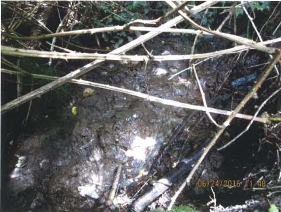
Photo 26. Looking upstream of stormwater drainage occurring along southern boundary of SE Briar Court development (PP16, Figure 5C)
