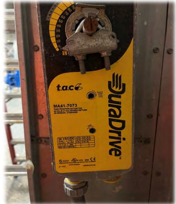
Second failed HVAC actuators in Headworks.
