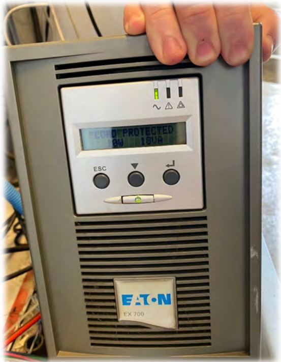
UPS that failed at Lift Station #3.
