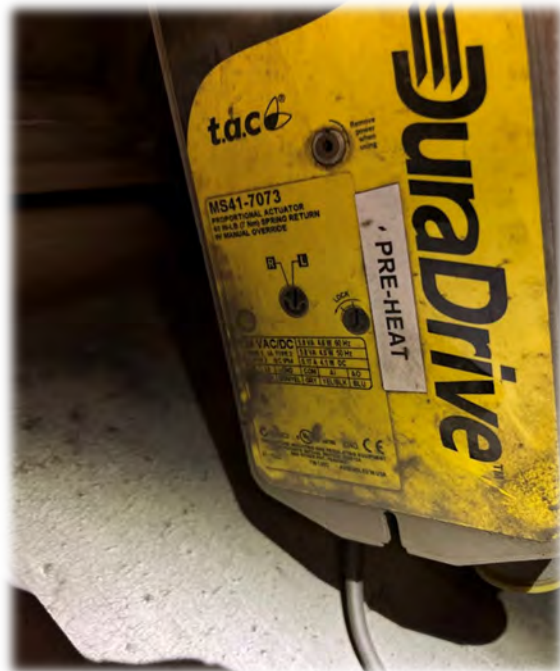
Failed HVAC actuators in the Headworks.
