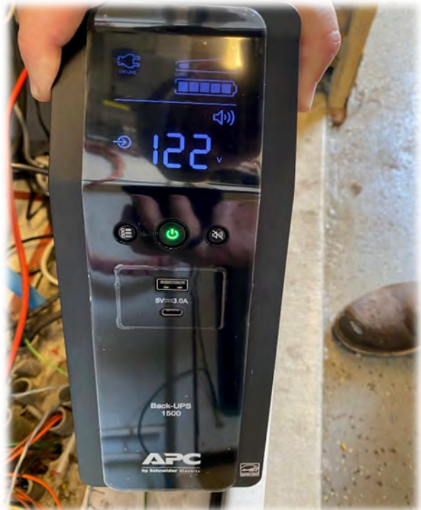
New UPS at Lift Station #3.
