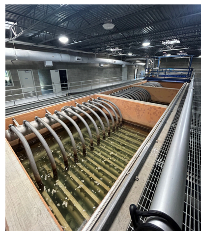
Membrane filters at the NCCWC treatment plant.
